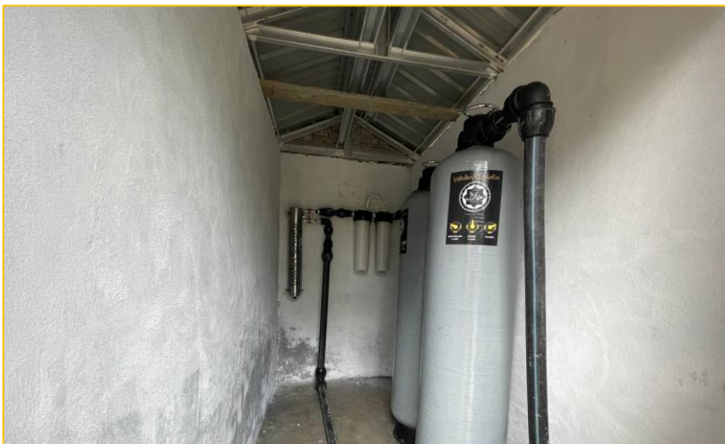
Membrane filtering system used to ensure that the water that reaches the homes of the villagers have been treated
