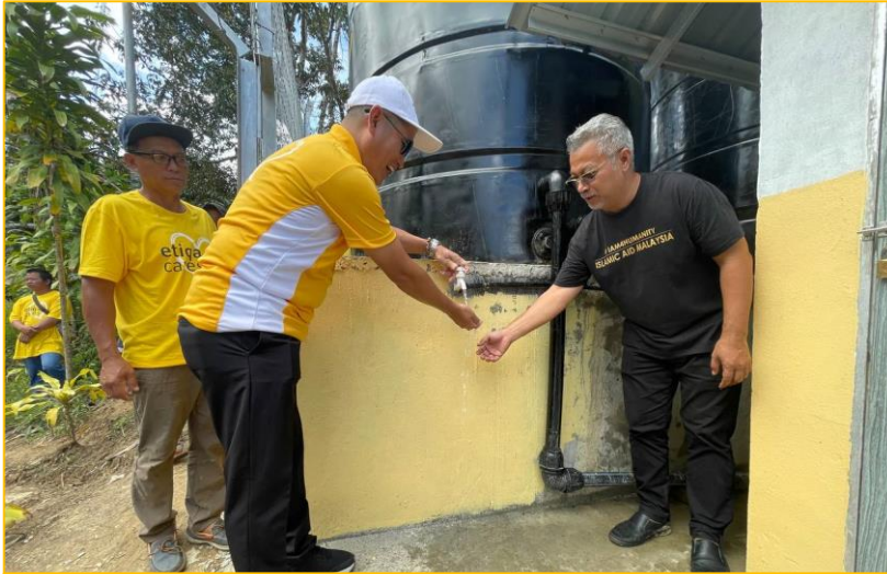
Aldo Kok, Regional CEO of Sabah Region, accompanied by Zawahir Abdullah, President of IAM, testing out the standpipes at the pumphouse
